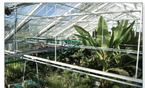
Tropical plants growing inside the greenhouse of the Solar Aquatics Wastewater Treatment have a key role in the water treatment process.
